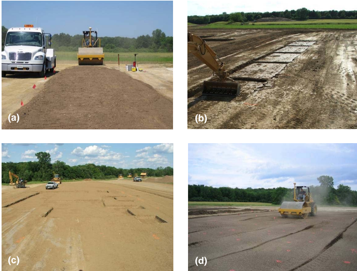
Figure 5.3. Construction and testing processes: (a) constructed test strip, (b) test Strip 1 excavations for variable lift thickness, (c) excavations for 510-mm lifts in spatial area, (d) compaction of spatial area
